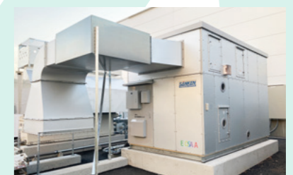
Example of implementation in a supermarket (outdoor unit)
